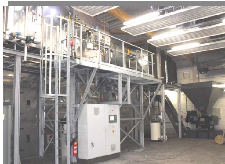
Control panel of the belt dryer
